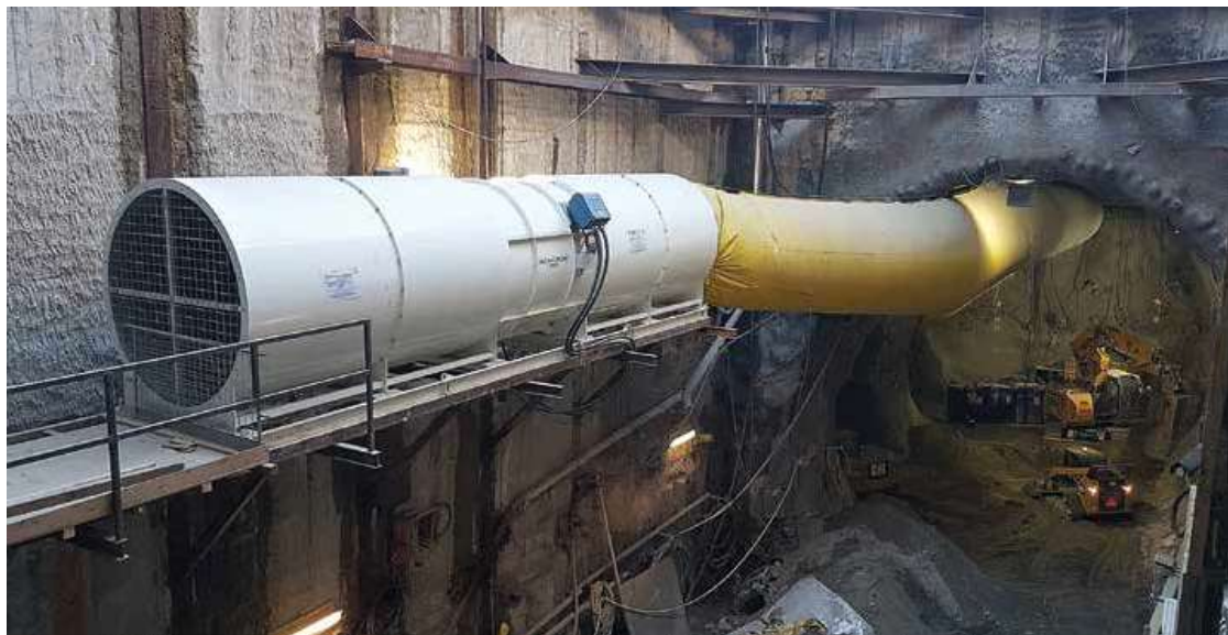
Schauburg Industries ducting in use at the Eglinton Crosstown Light Rapid Transit (LRT) project in Toronto.
